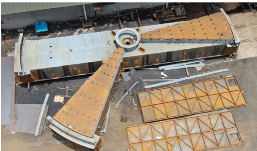
TYPE OF JOB - Tri-Sector Plate Assembly Industry – Power Plant HEIGHT AND Width – 2.5 M Height and 16 Meter length, 4 meter width in dismantled condition WEIGHT - 60 MT approx
